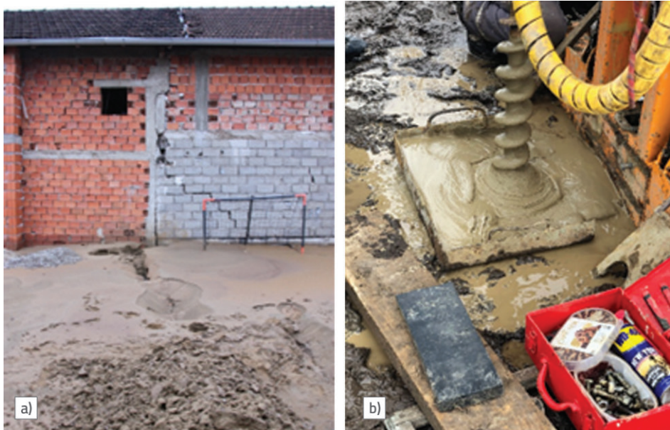
Figure 1. Evidence of soil liquefaction in the village of Brest Pokupski: a) sand ejecta and surface cracks, b) saturated sand deposits
